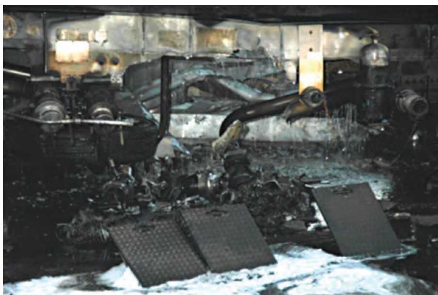
Figure 19 Fill point area after the fire was extinguished with metal covers in the open position [photograph courtesy of FESA]
