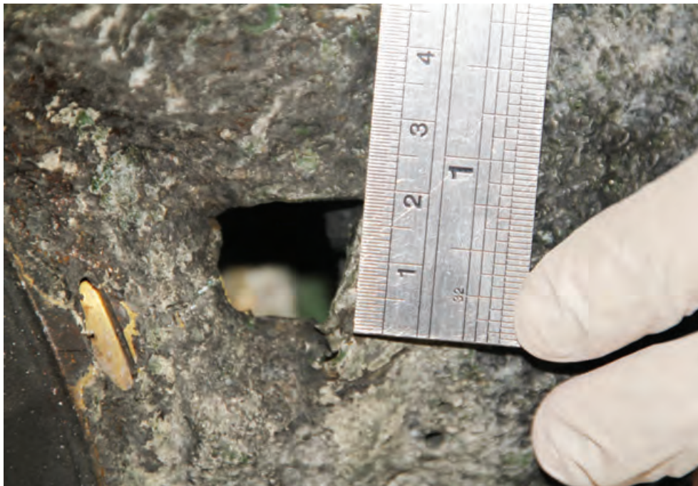
Figure 40 Close up of hole in vapour recovery elbow pipe
