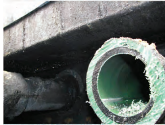
Figure 47 Tank 2 fill pipe inside containment sump — fill pipe is fire affected
