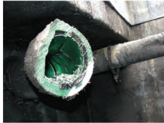
Figure 53 Tank 4 fill pipe inside containment sump — fill pipe is partially fire affected
