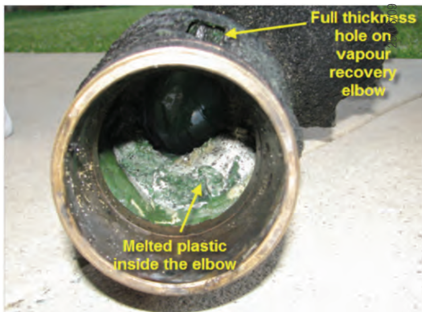
Figure 38 Top section of vapour recovery elbow pipe, the hole in the elbow and melted plastic inside the pipe
