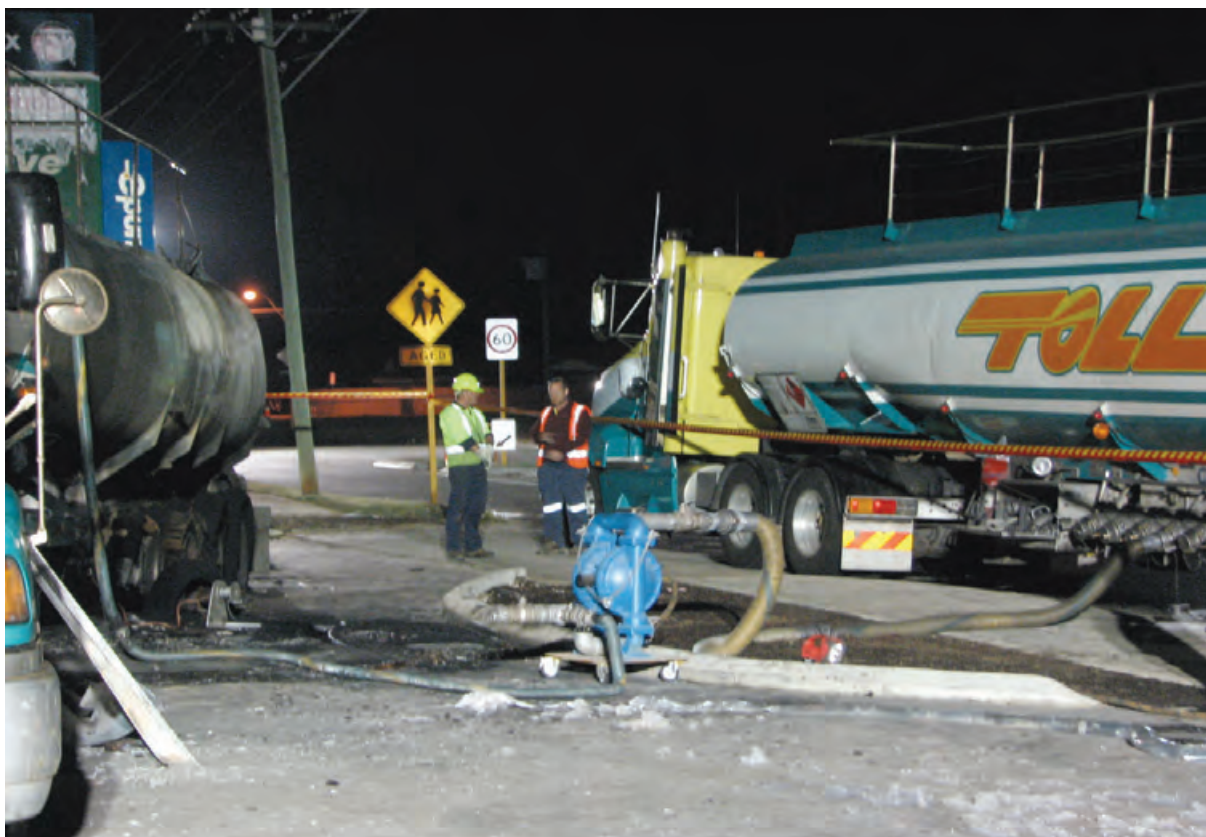
Figure 21 Transfer of fuel to the recovery tanker using an air-operated diaphragm pump
