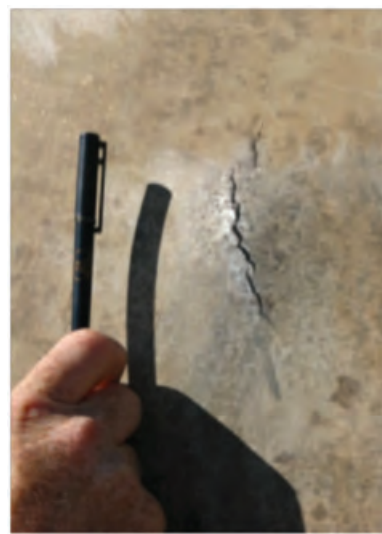
Figure 31 Fine crack on the tank shell of compartment 6 (passenger side)
