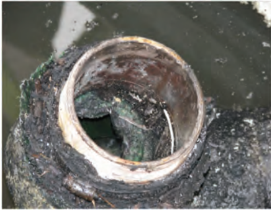
Figure 46 Fill point opening of tank 2 — significant melting of green plastic pipe
