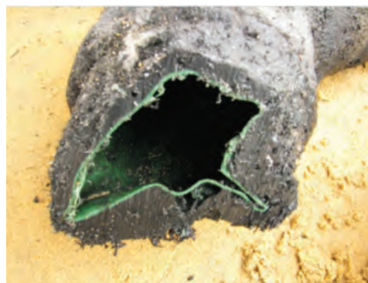
Figure 50 Deformed fill pipe elbow of tank 3 after it was cut from the fill pipe
