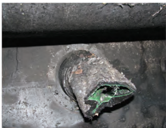
Figure 49 Tank 3 fill pipe inside containment sump — fill pipe is significantly fire affected
