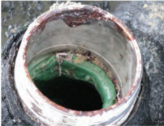
Figure 52 Fill point opening of tank 4 — noticeable melting of green plastic pipe
